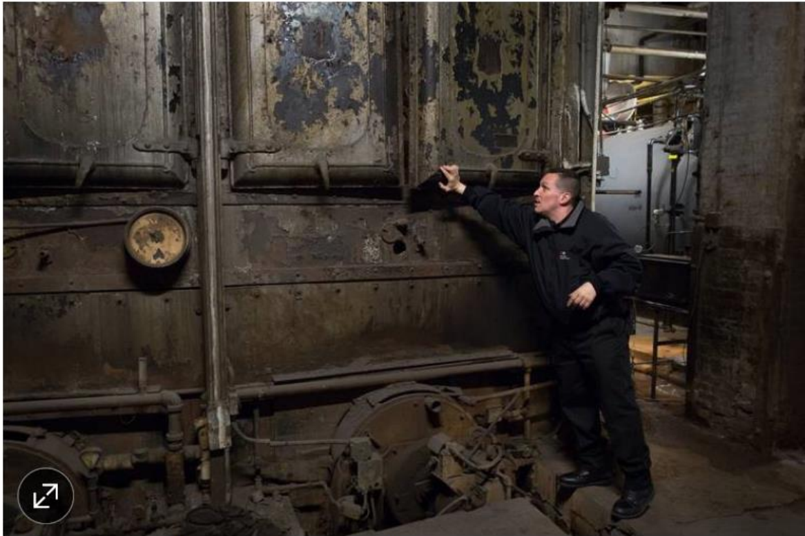
Superintendent Sunny Atis in the boiler room of the Flatiron Building. PHOTO: AGATON STROM FOR THE WALL STREET JOURNAL
